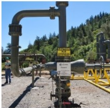
Injection Well (photo: KQEDQuest)
